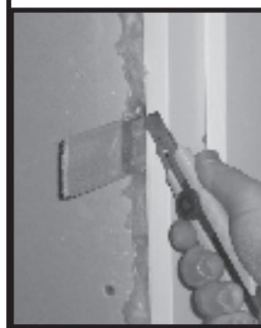
Figure 11 (left): Insulate between the jambs and the wall studs all around the door.
