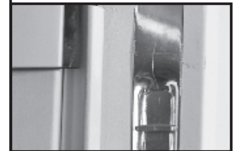
Figure 5: Correct sagging until the flush bolt slides freely into the pre-drilled hole (not typical of most units) in the head/threshold.
