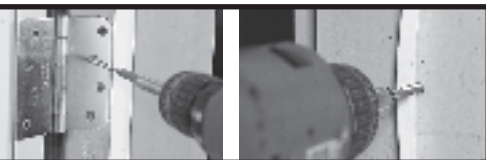
Figure 7 and 8: The second set of supplied screws is installed in the vacant hinge holes or under the weatherstripping.
